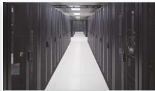
Control Room / Data Center
