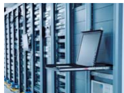
Control Room/ Data Center
