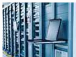
Control Room/ Data Center
